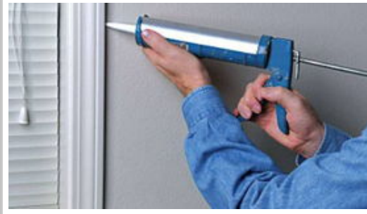
Air leakage at window casements and typical solution:
