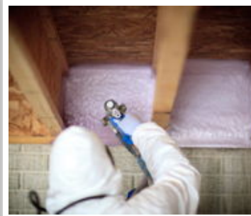
Spray Foam solution to uninsulated and leaky box sill:
