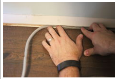
Air leakage at baseboards and typical solution:
